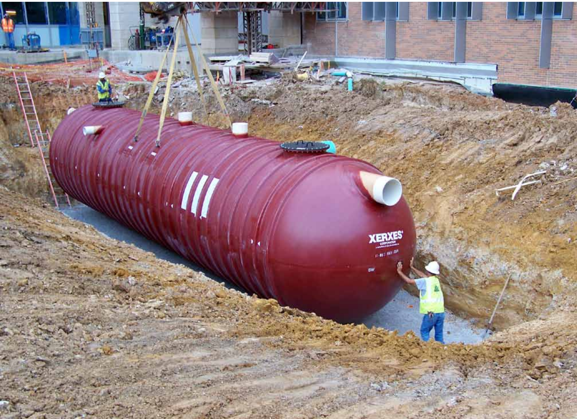
Rainwater/stormwater collection tank at the University of Texas-Arlington.
